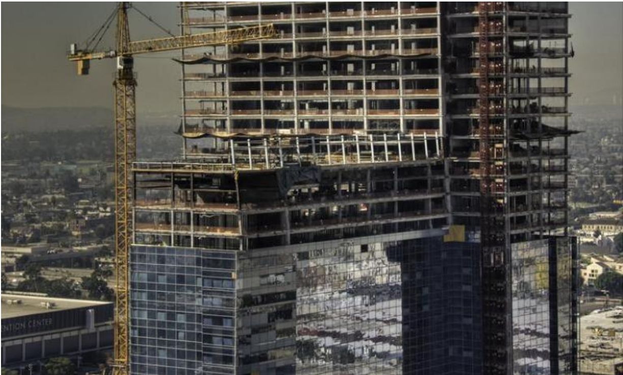
FIGURE 1-3: L.A. LIVE TOWER AND RESIDENCES, LOS ANGELES, CA (IMAGE COURTESY OF © 2015 ENCLOS CORP)
