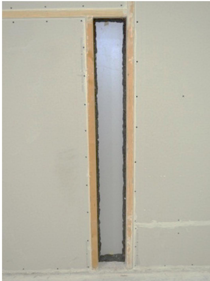
FIGURE 4-7: ELEVATION OF THE MULLION IN THE FILLER WALL WITH SEALED PUTTY PERIMETER
