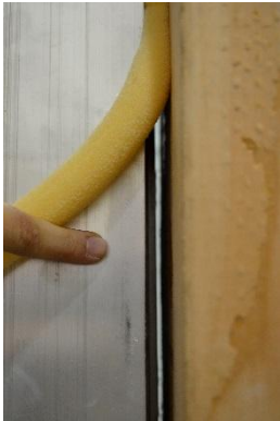
FIGURE 4-5: A 1/4" GAP BETWEEN MULLION PERIMETER AND FILLER WALL
