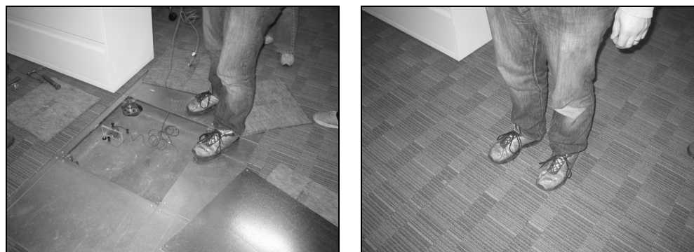
Figure C.9 Unintrusive installation of a vibration transducer underneath a false floor for long term monitoring.
