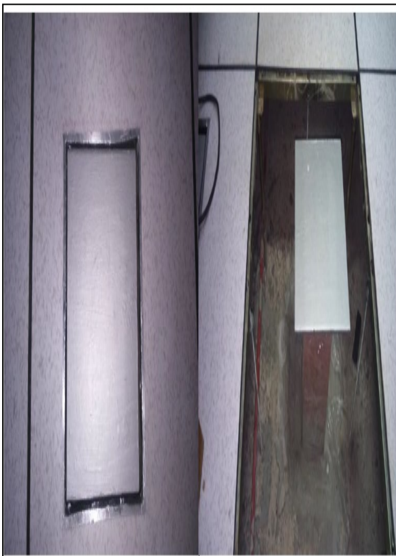
Figure 3 : Shows the suggested steel base mounted from the concrete to the raised floor at Lab.1. (Dimension of steel base is: length=250mm , width=250mm & height = 300mm.)
