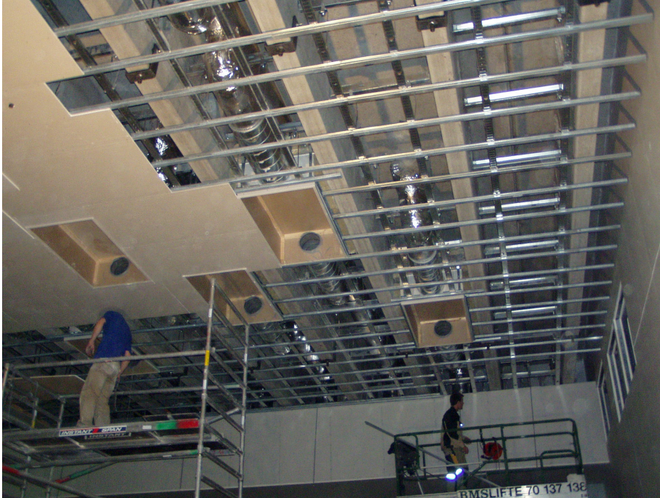
Figure 5. Photo of the sound insulating ceiling used in the Rhythmic Hall with supplementary measures for incorporating ventilation diffusers.
