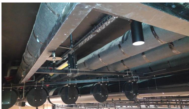
Figure 4 – Rotating cylinders on the ceiling (lower part of the figure) for changeable acoustics.
