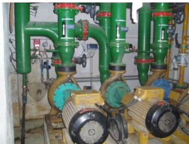
Figure 5 : Pompes chaufferie – Fixations rigides
