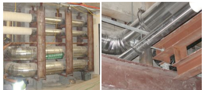
Fig. 6. Vibration Isolated Pipe Racks.
